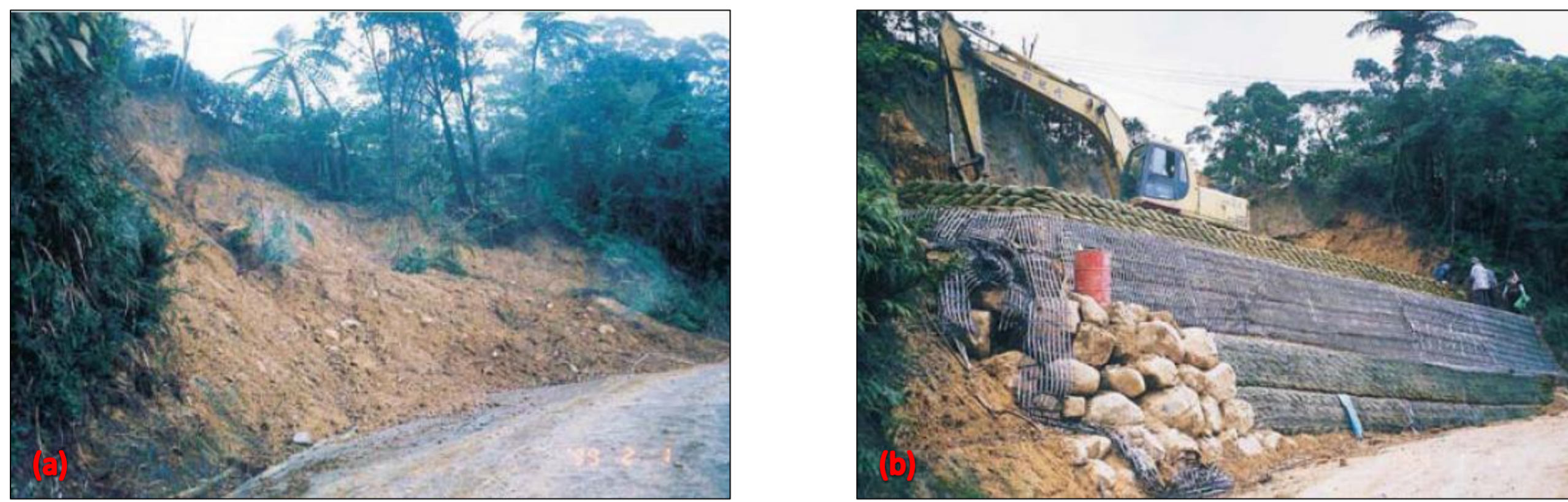
Figure 1: (a) Failed slope (b) reconstructed slope using reinforcement-drainage geocomposite and backfilled with original soil
